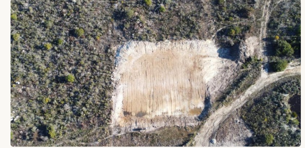
Topographic survey – building footprint positioned within the reserve contours via engineering survey
