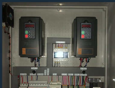
VSD and PLC panel — pressure, flow and performance management
