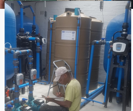
Field technician completing maintenance and inspection log on site – structured O&M records maintained across all facilities
