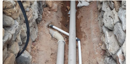
Utility trench coordinating water, drainage and electrical routes beneath stone retaining walls
